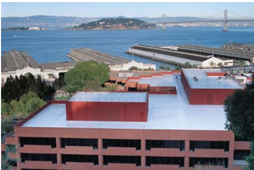
A Flex roofing system on a prestigious office building overlooking San Francisco Bay resists high moisture and salt air conditions.
